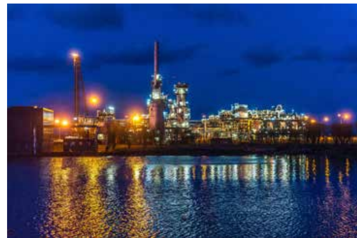
St Fergus Terminal, United Kingdom. Photo credit: North Sea Midstream Partners (NSMP).
